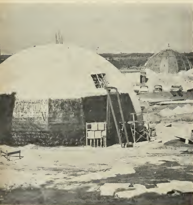
MINUTEMAN'S two concrete-shell blockhouses, left, will be covered with sandbags for extra protection. Assembly and fuel storage facilities are being built elsewhere on the Cape.
