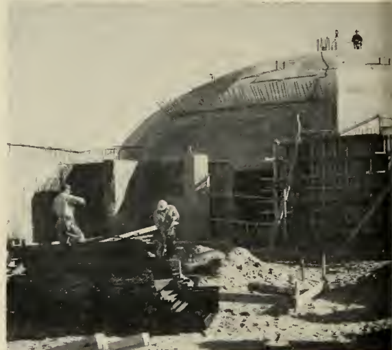
GRANDDADDY of them all, Saturn will have the largest service tower on the Cape—rising 305 feet off the ground. Contracts for blockhouse and other facilities total $10 million.
