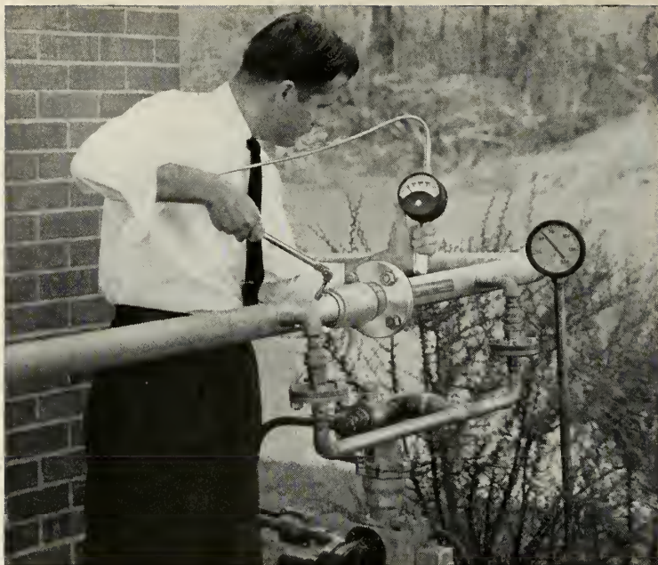
CEC Transfer Line installation shows temperature of outside pipe only 2°F. different from ambient.
