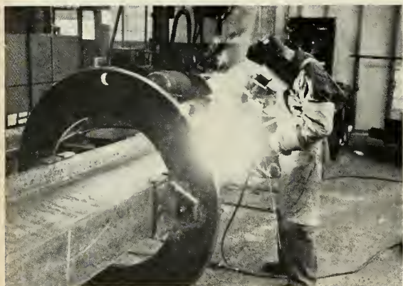
1 Beams supplied by U.S. Steel are cut to length and webs reinforced in first operation of launcher base fabrication.
