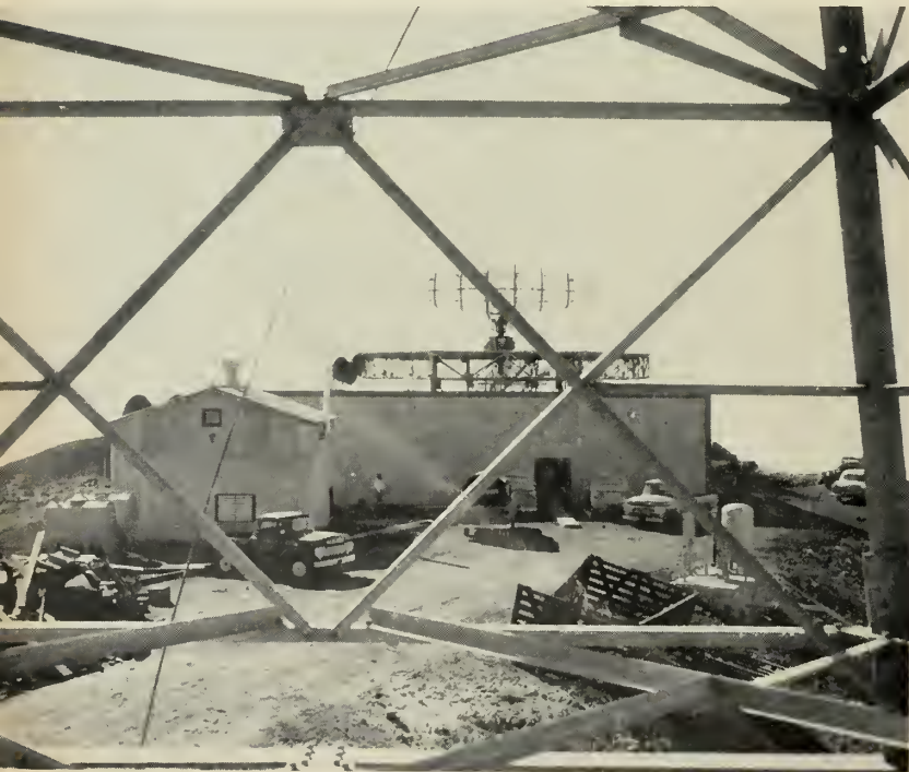
REMOTE RADAR building under construction at Point Arguello. Wild deer are frequently spotted watching as workmen unload electronic equipment.
