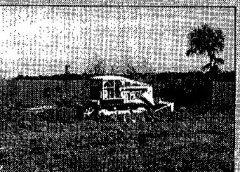
Workers begin to build the Manned Spacecraft Center in Clear Lake. Page 6
