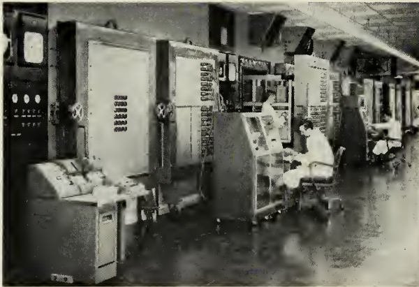
A ROW OF Inland's environmental chambers with automation equipment in front of doors. Accuracy is closely checked.
