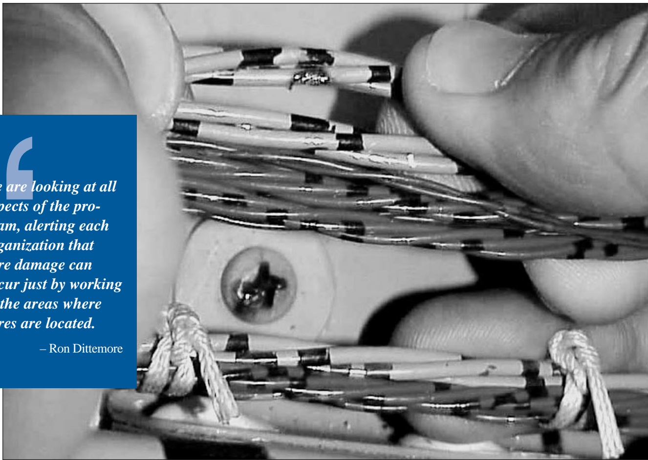
KENNEDY SPACE CENTER, FLORIDA – A wire damaged by abrasion from the head of a screw (seen below the bundle) was found during electrical wiring inspections in Columbia's payload bay. During launch of Columbia on mission STS-93, a damaged wire caused a short circuit in two separate main engine controllers.
